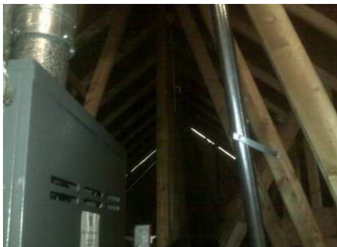
Fig. 5 Attic shot, can't see it but center of dipole is up there. Notice my furnace right near by!
